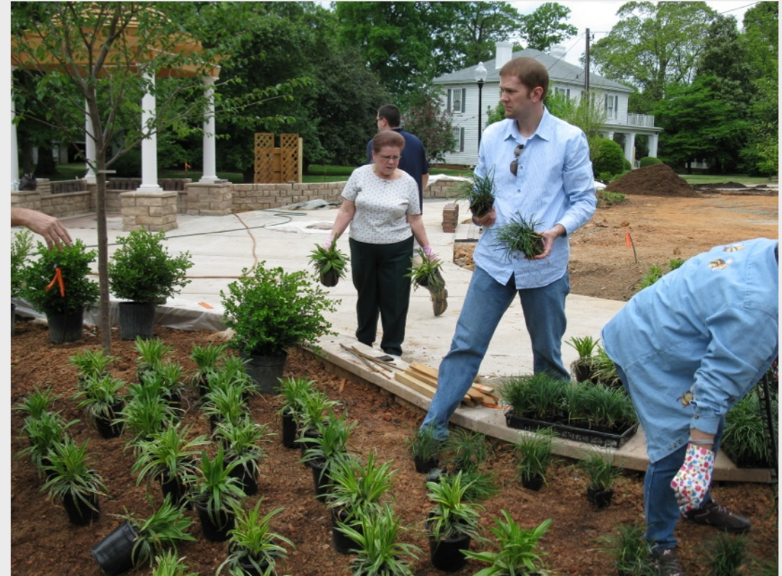
Residents and Town of Matthews employees complete landscaping for the town's new pocket park. (Photo Credit: Town of Matthews)
